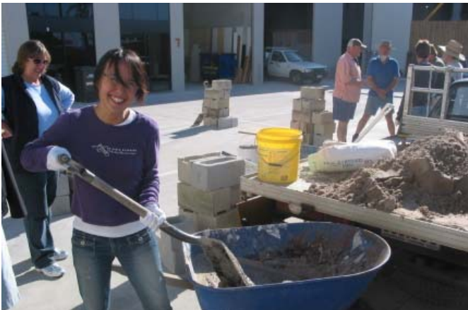
Construction team from Harvest City Church on the Gold Coast - learning to lay blocks
