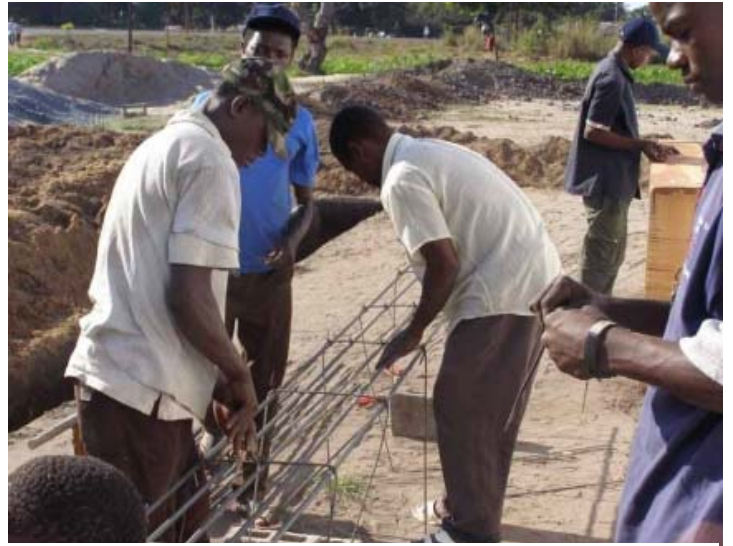
Steel boxing for the classroom footings being built by the Mozambican team.
