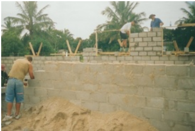
Blake working on the wall that collapsed when a load of sand was unloaded on it
